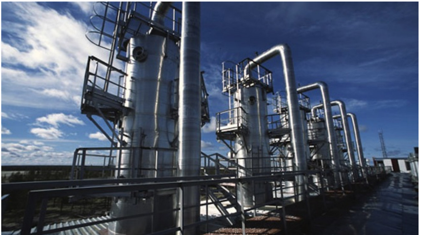
A Novatek facility
